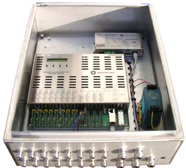
Fig. 1: DDAU II –shown in its IP66 enclosure in connection with the WEB Server and Power Supply
